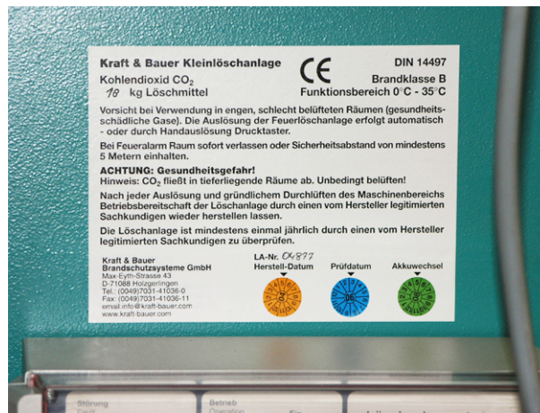
Example: Inspection stickers Kraft & Bauer
